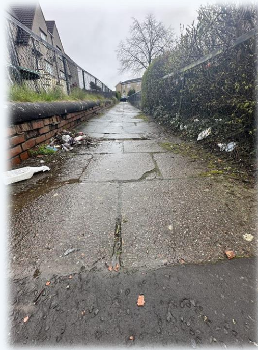
Pathway at Loreny Drive is uneven – Choice Places is looking into having this re-levelled.
