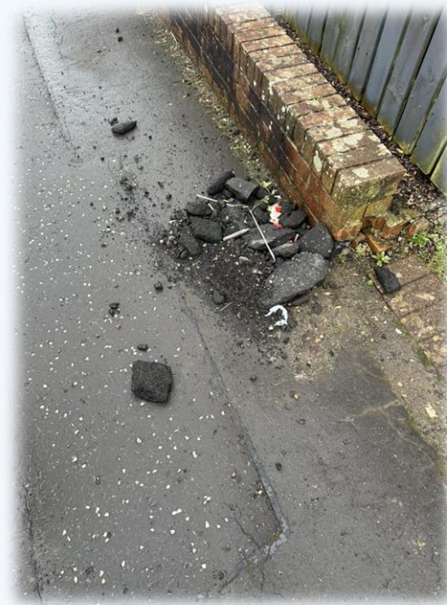
Rubble from tarmac on public footpath will be reported to East Ayrshire Council as this is a potential trip hazard.
